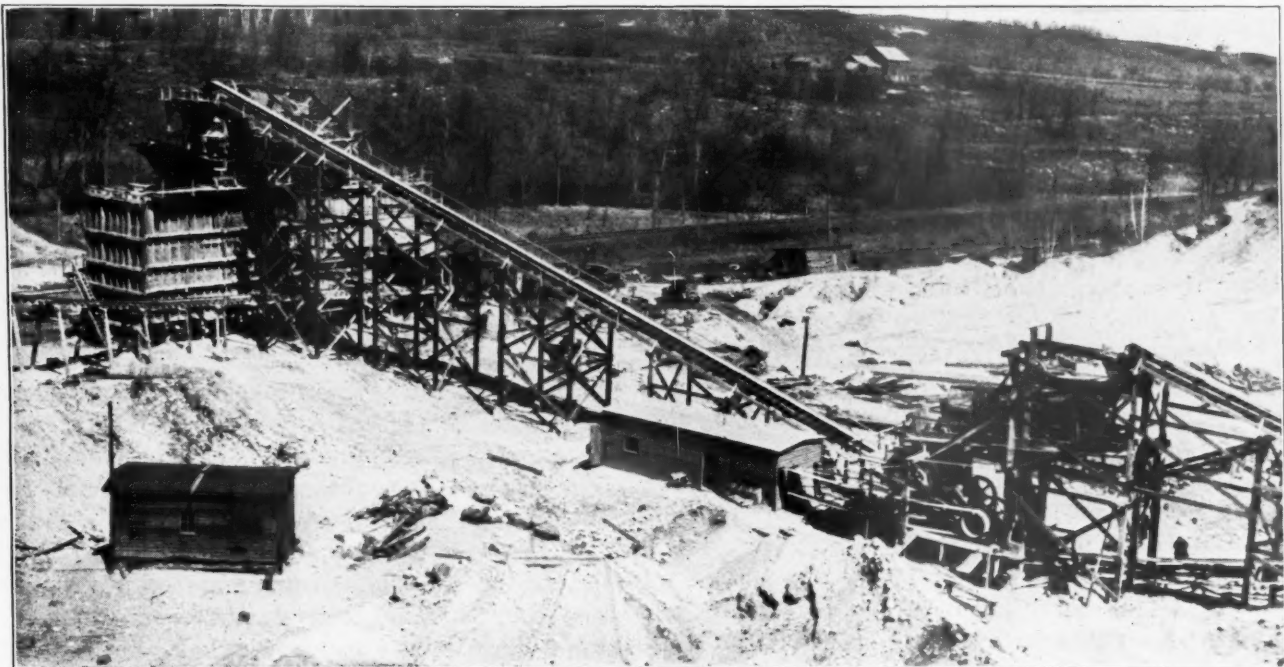
Crushing Plant Is at Right and Material Is Taken by the Long Conveyor to the Screening and Storage Unit at Left.
